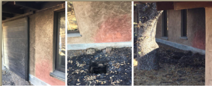
Fig. 2. Norrbon Road - Mineral oxides in Natural Hydraulic Lime turn pink when heated.
