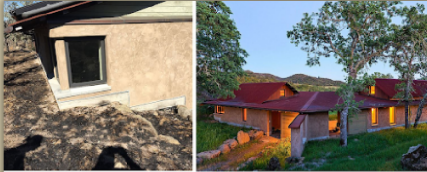
Fig.1. Norrbon Road Strawbale Home - fires burned to the foundation on but not up the walls.
